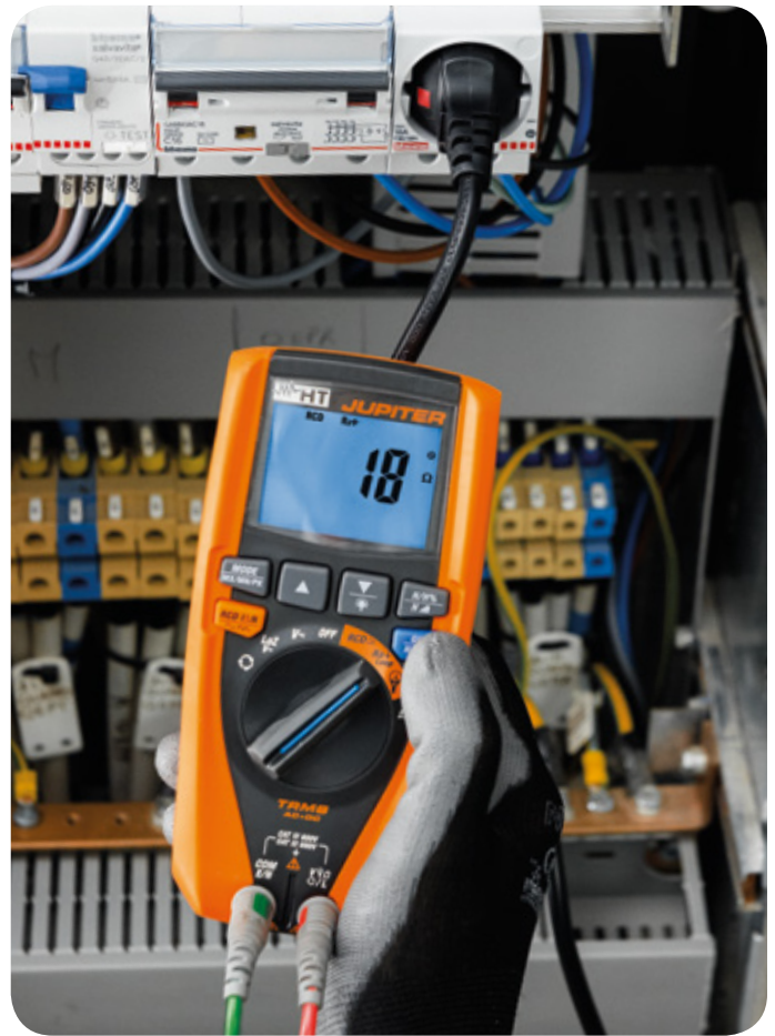
Non-trip earth ground resistance measurement.
