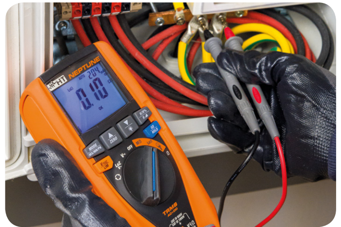
Continuity of protective conductors .
