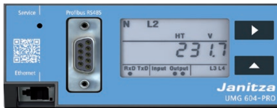
Fig. Front view of UMG 604 -PRO control element
